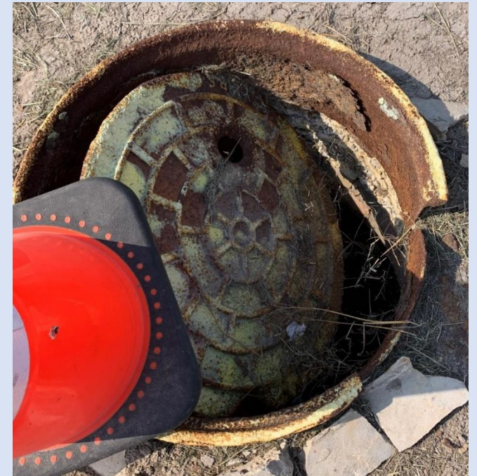
Recent photo of Iron Cover Dropping into Corroded Iron Frame
