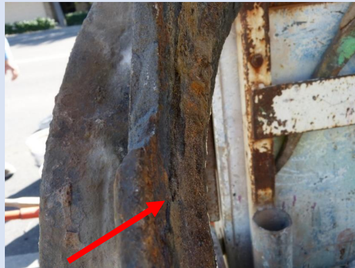
The seat for the cover is completely degraded and the frame ID is flush. The Cover is virtually riding on air!
